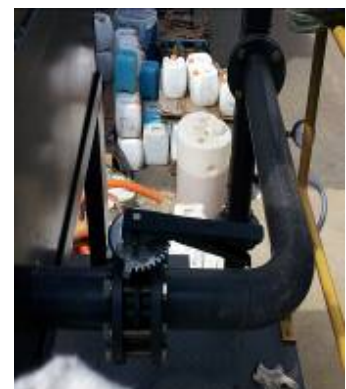
Flow control valve
