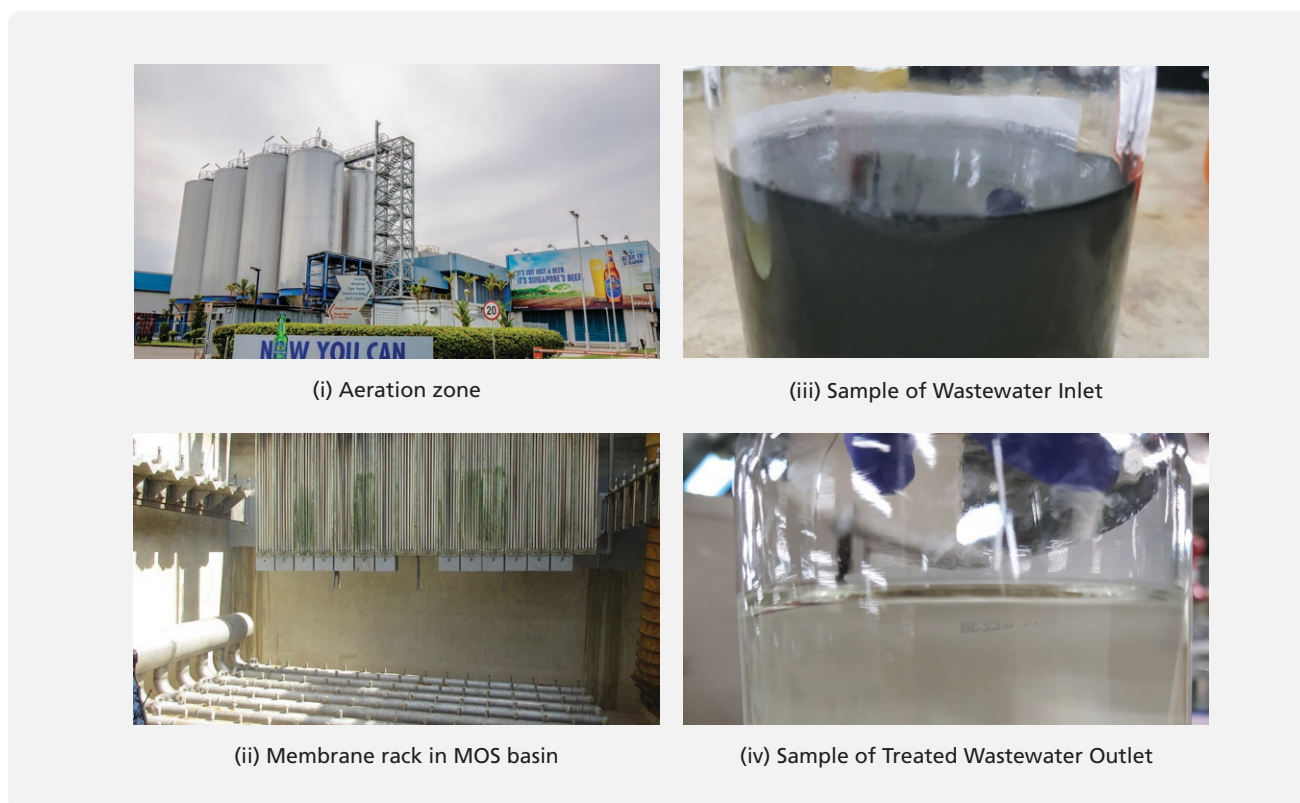
Figure 6: Pictures of (i) Aeration Zone (ii) MOS Basin (iii) Wastewater Inlet (iv) Wastewater Outlet
