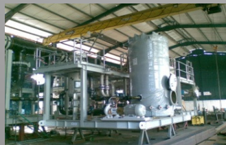
Sea Water Pre-treatment Unit
