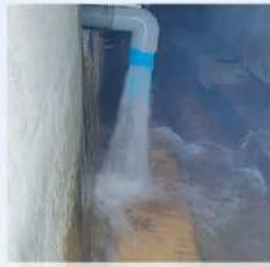
Snapshot of water discharge
