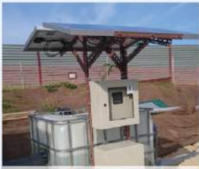
Solar-powered TSS system
