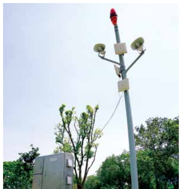
Fig 5.2 A safety node with warning lights at Kallang River at Bishan-Ang Mo Kio Park.
