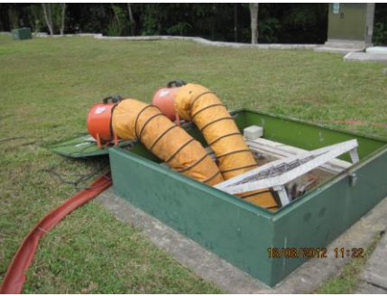
Lighting & Air blower
