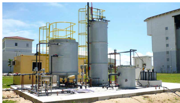
Fig. 2: DEMON® pilot plant at Changi Water Reclamation Plant (WRP)
