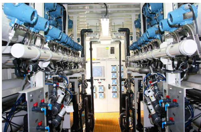
Fig. 2: The two parallel RO trains in the pilot skid, complete with process control and instrumentation monitoring
