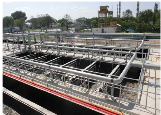
Fig. 2: The UASB-CMBR demonstration plant at Jurong Water Reclamation Plant
