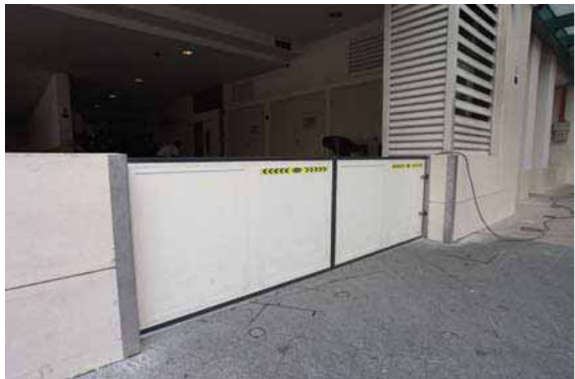
Figure 6.2.5 Swing-type flood barrier in open (top) and closed (bottom) positions at access to loading/unloading areas.
