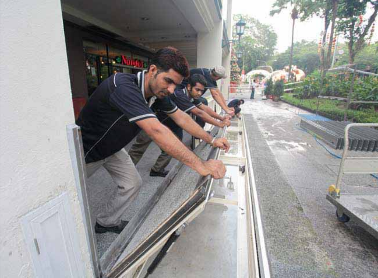
Figure 5.7 Regular tests and inspections of flood barrier systems are necessary to ensure that the system can be reliably activated during flood events.
