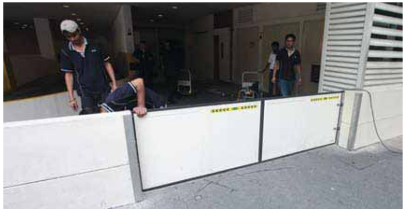
Figure 4.14 Manually operated swing-type barrier system.
