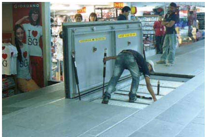
Figure 4.12 Maintenance staff checking and testing a flip-up flood barrier.
