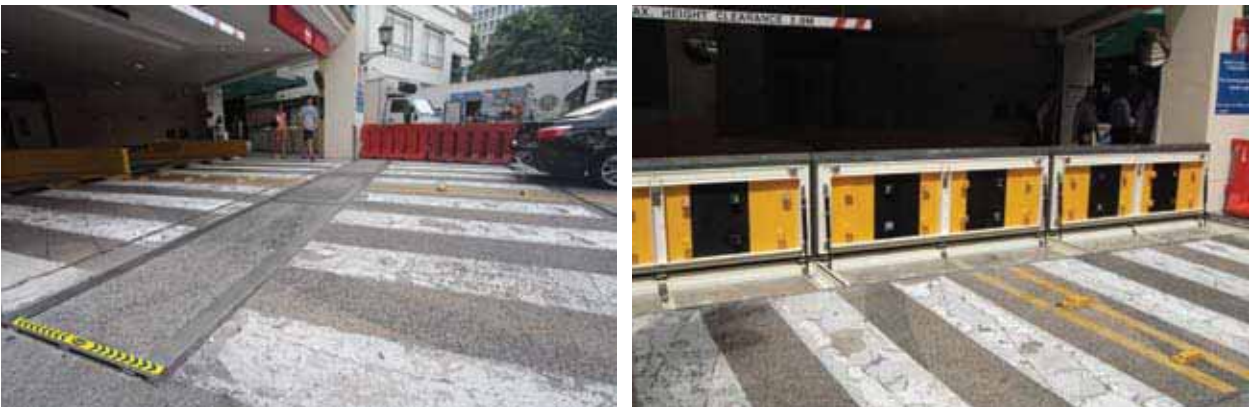
Figure 6.2.3 A flip-up barrier at the entrance to the basement carpark in closed (left) and open (right) positions.
