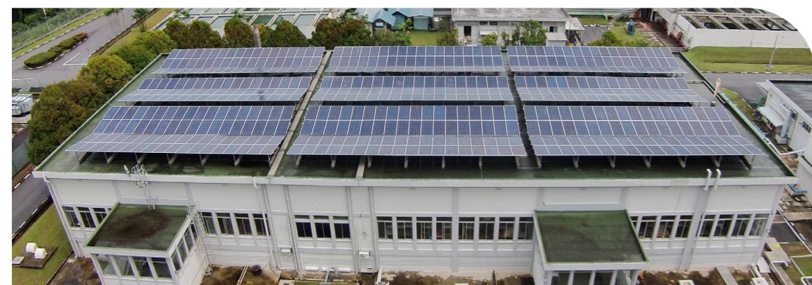
Rooftop solar PV system at Choa Chu Kang Waterworks.
