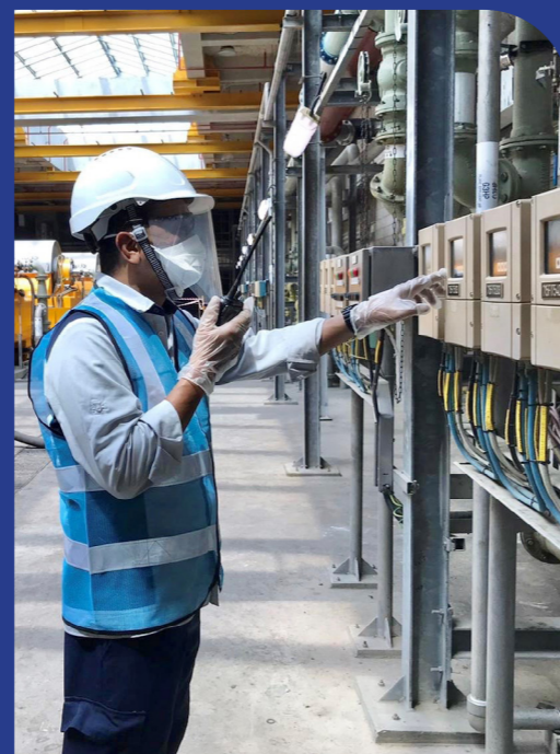
PUB officer at Changi Water Reclamation Plant working during the COVID-19 pandemic.
