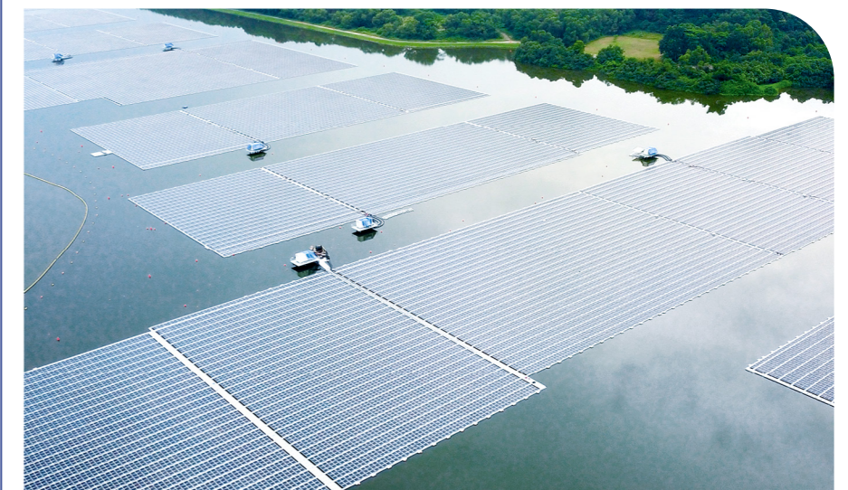
Aerial view of Tengeh Floating Solar Farm. (Photo credit: Sembcorp Industries)
