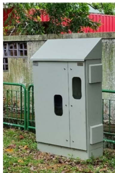
VOC Monitoring Unit
