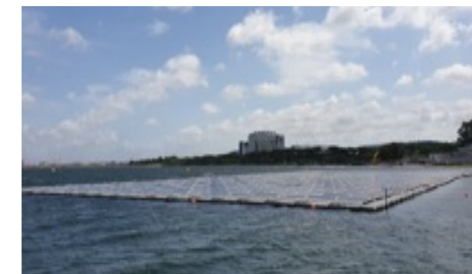
1.5 MWp system at Lower Seletar Reservoir
