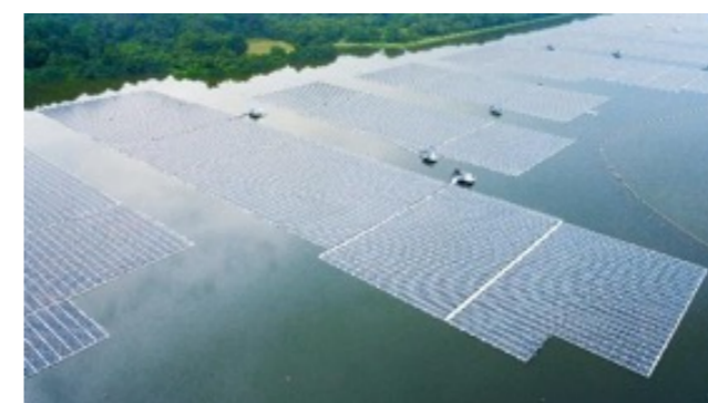
60 MWp system at Tengeh Reservoir
