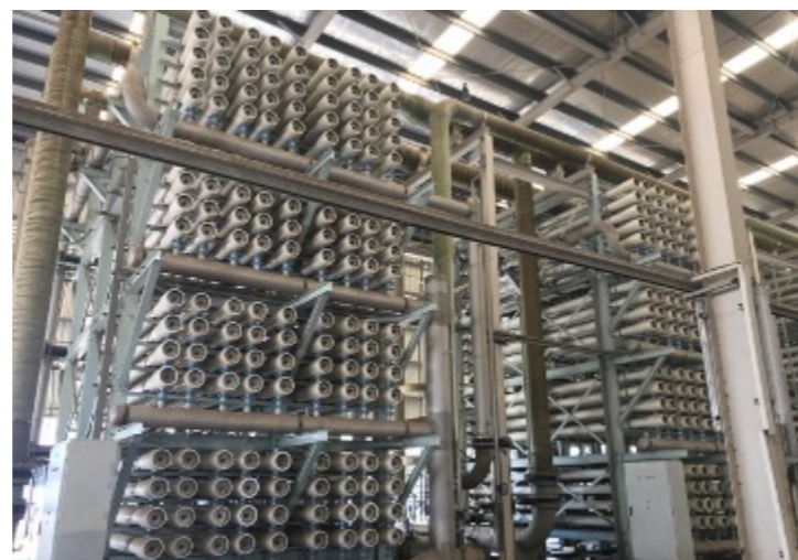
Chestnut Avenue Waterworks commissioned 26 new trains of Reverse Osmosis Membrane
