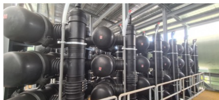
Enhanced water treatment with 14 new trains of Disc Filters at Chestnut Avenue Waterworks
