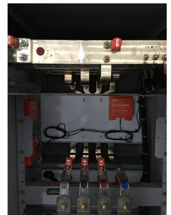
Exertherm Sensor Cable in Hotspot Temperature Monitoring System
