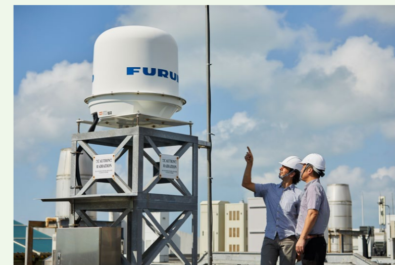
Radar at Changi Water Reclamation Plant
