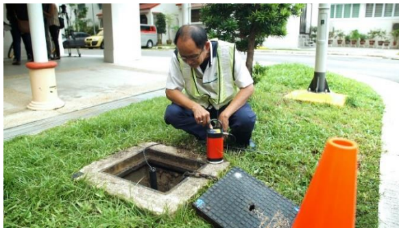
PUB technicians carrying out leak detection inspection work using leak noise loggers and correlators
