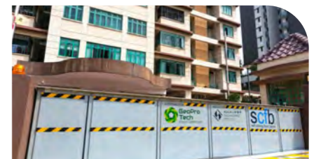
Automatic Flood Barrier at Fortune Park Condo.
