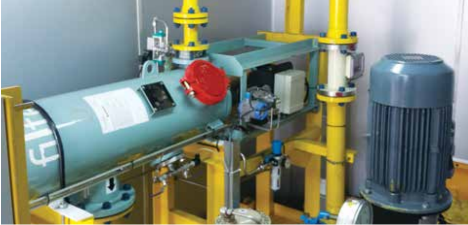
Fig. 1: Pilot unit at the pumping station in Kranji
