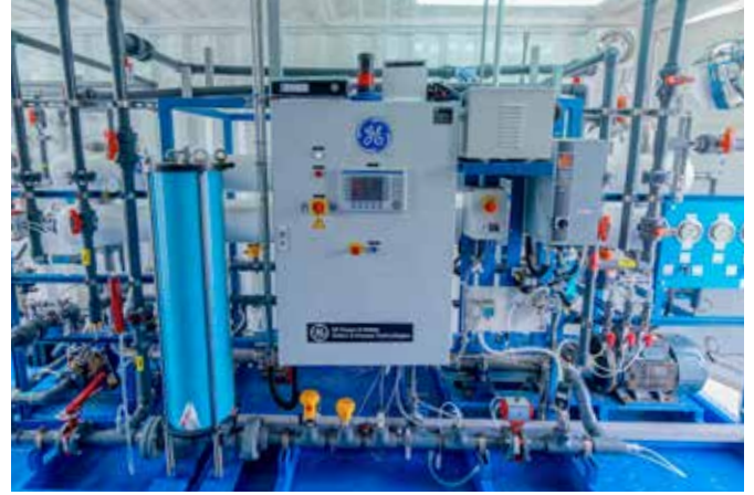
Fig. 2: Pilot-scale demonstration set up at PUB's R&D testing facility in Tuas
