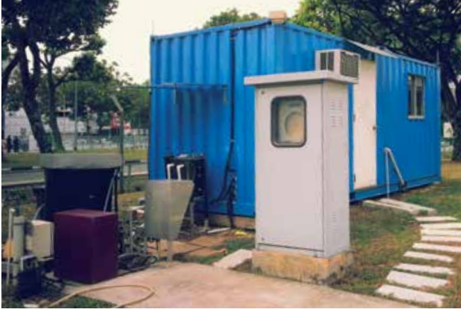
Fig. 1: MES system installed at Tanjong Penjuru Pumping Station for the field trial
