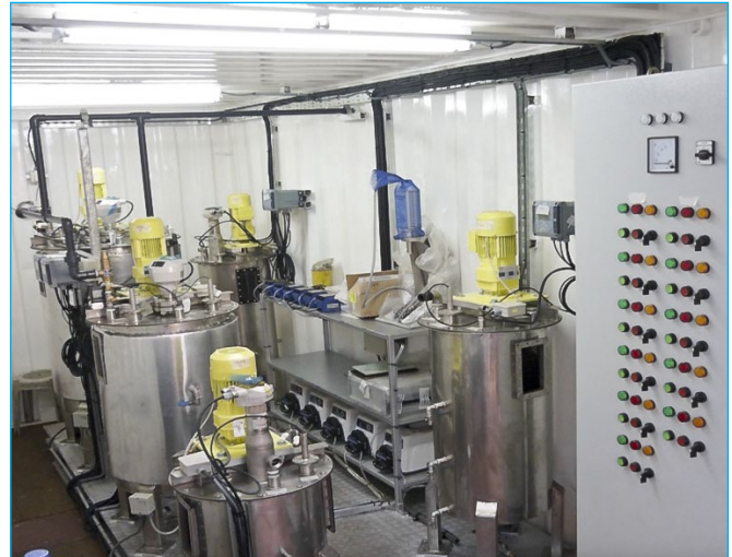
Fig. 2: The sludge biodigestion pilot plant
