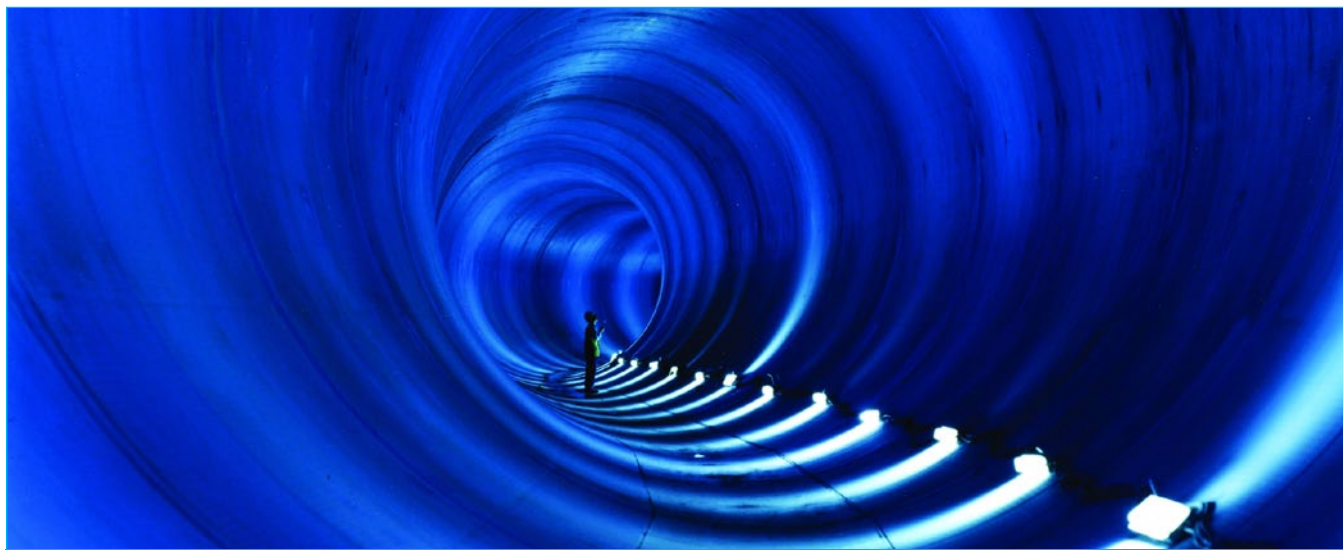
Fig. 1: The six-meter Deep Tunnel Sewerage System where the RMSI is employed for inspection
