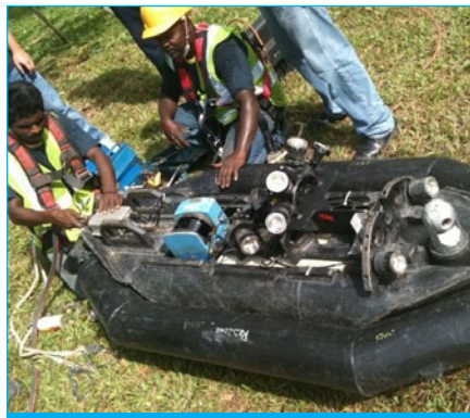
Fig. 2: Modified Raft Inspection Platform is used for inspection when the water level in DTSS is high
