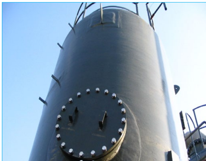
Fig. 1: A view of the biocarbon tower that is removing sewage gas odours at the Kranji Water Reclamation Plant
