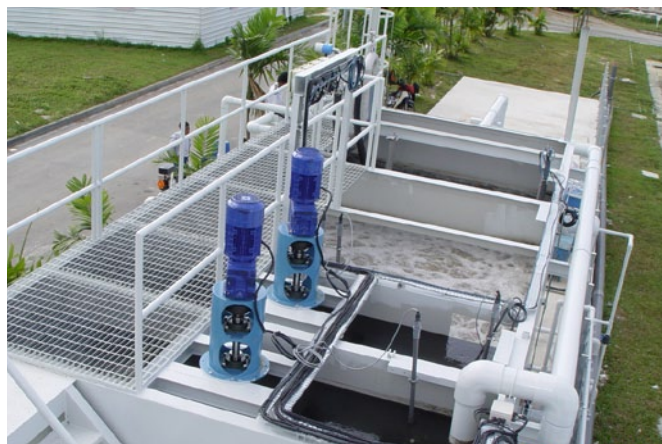
Fig. 1: One of three pilot membrane bioreactor pilot units installed at Bedok Water Reclamation Plant in 2003
