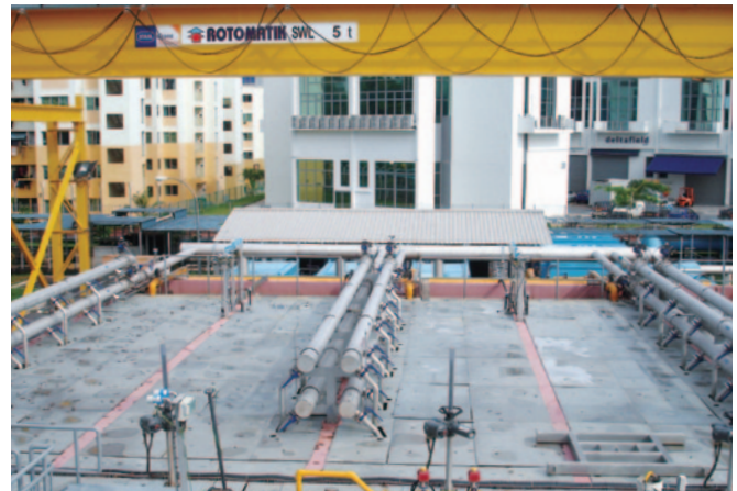
Fig. 3: At Ulu Pandan, PUB scientists and engineers oversaw the construction of an MBR tank suitable for processing up to 23,000 m 3 of wastewater per day. From Ref. 3 (© 2008 IWA).
