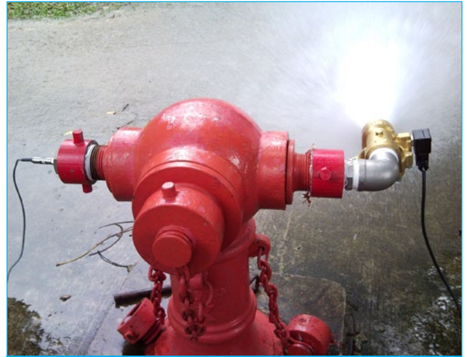
Fig. 2: Emulation of a burst water main was quickly detected by a neighbouring sensor node of Singapore's prototype monitoring network
