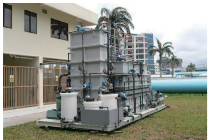
Fig. 5: A miniature pilot MBR plant constructed at the Ulu Pandan facility to test a new membrane module design. From Ref. 4 (© 2009 IWA).
