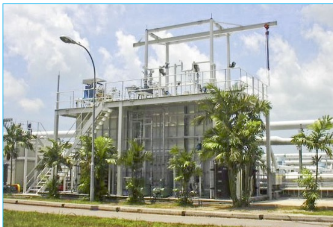
Fig. 2: The new membrane bioreactor system test-bedded at the Ulu Pandan Water Reclamation Plant
