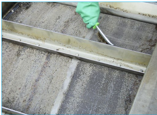
Fig. 1: The left side of this rotating drum screen is almost completely blocked with debris, and so needs to be cleaned
