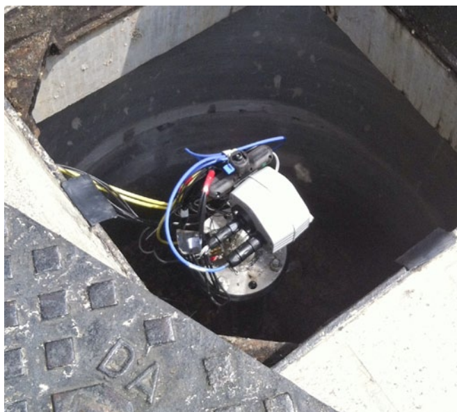
Fig. 4: The incorporation of a well-calibrated hydraulic model allows study of physical properties of the distribution system
