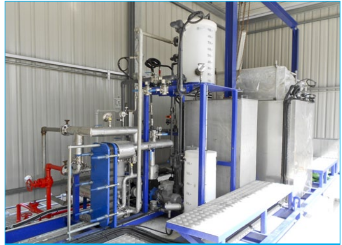
Fig. 2: Testing the membrane distillation bioreactor for treating used water in a pilot plant installed at an oil refinery
