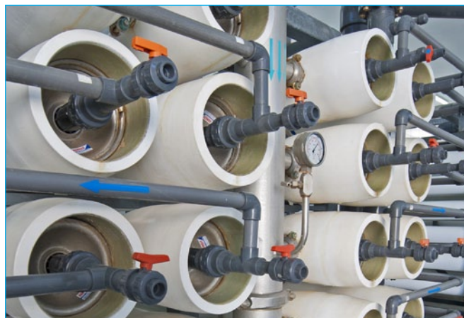
Fig. 2: Rising pressure in filtration systems can indicate biofilm formation, but such warnings often arrive too late to prevent serious contamination
