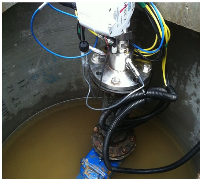
Fig. 3: Insertion probes detect anomalies at various points throughout the water distribution system
